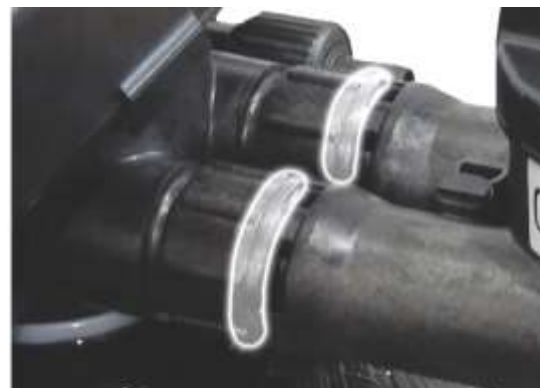
11b (Connected Properly)
